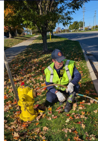
FIREFIGHTER KEVIN JONES - HYDRANT PUMPING FOR WINTER TO PREVENT WATER FREEZING
